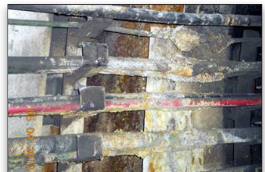
Original tunnel lining installed in the 1970s showed signs of water ingress, causing potentially unsafe conditions.
